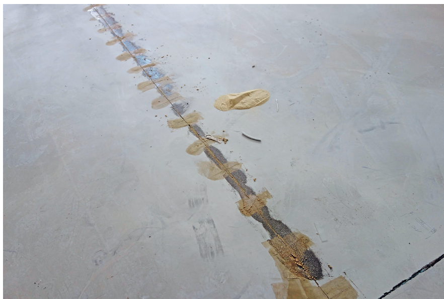
Kraftschlüssig verharzte Scheinfuge.
